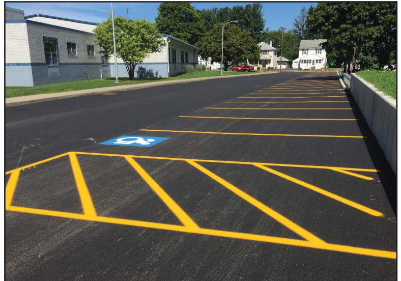
New sidewalks, retaining wall, and parking lots are complete at Charles F. Johnson.
