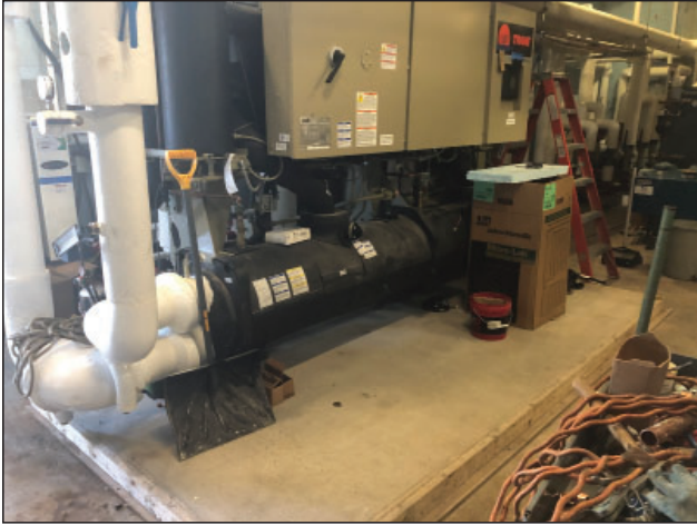
New chiller installed at CFJ for building wide air conditioning.
