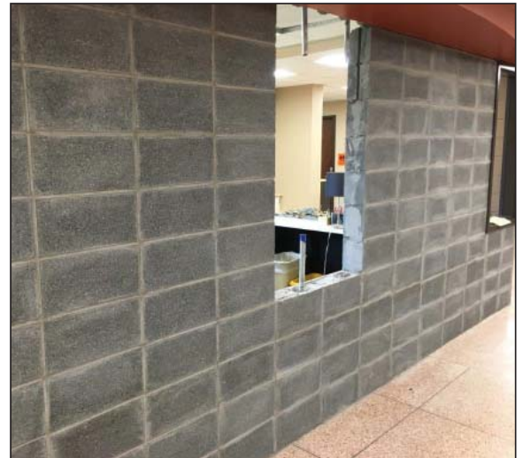
Additional windows from the main office into the corridor are being installed at AGM and TJ Watson.
