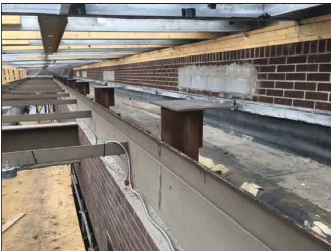
The structural steel support is in place for the new High School skylight.
