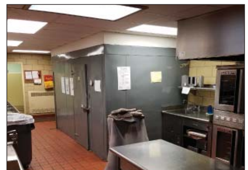
The walk-in cooler/freezer will be replaced at Thomas J. Watson.
