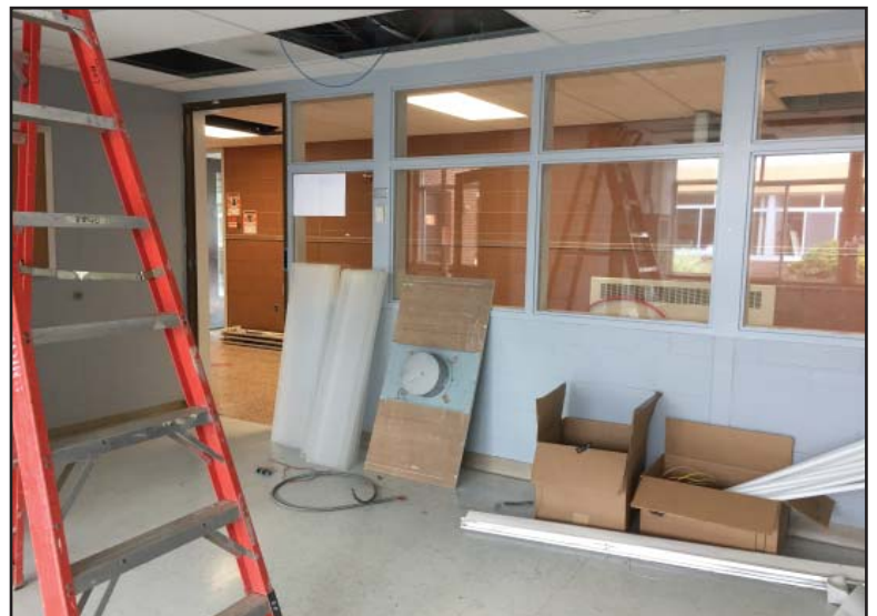
Demolition has begun at AGM for the new secure vestibule and main office.
